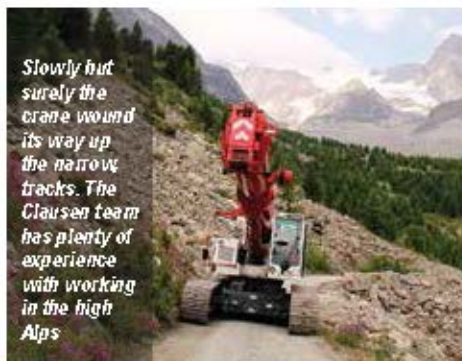
The mountain station for the new Hörnli/Hörnli chairlift is being built at the foot of the Matterhorn. The LTR 1060 overcame steep gradients to get to the site
